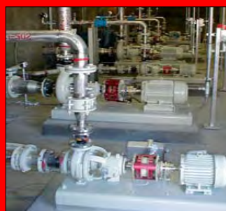
11 ASD's at Ashland Water Treatment Plant in Oregon
