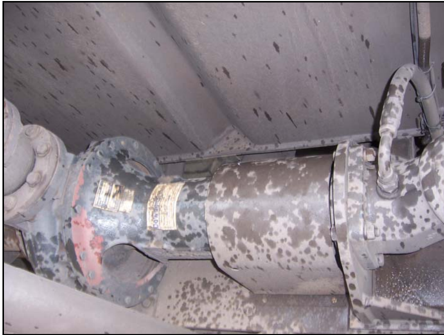
Figure 1 Before MagnaDrive- Pumps failed due to alignment issues
